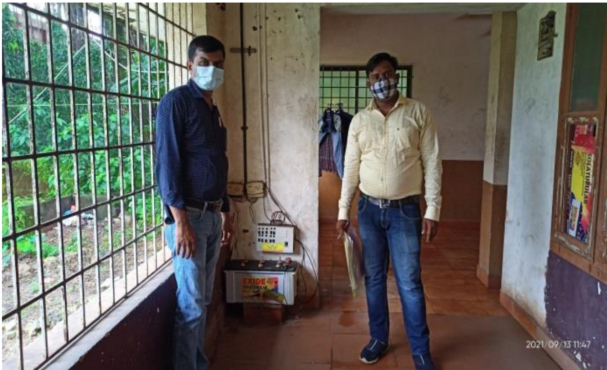
Provision of Solar Light battery
