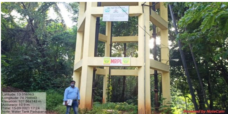
Padupanambur Village Water overhead tank
