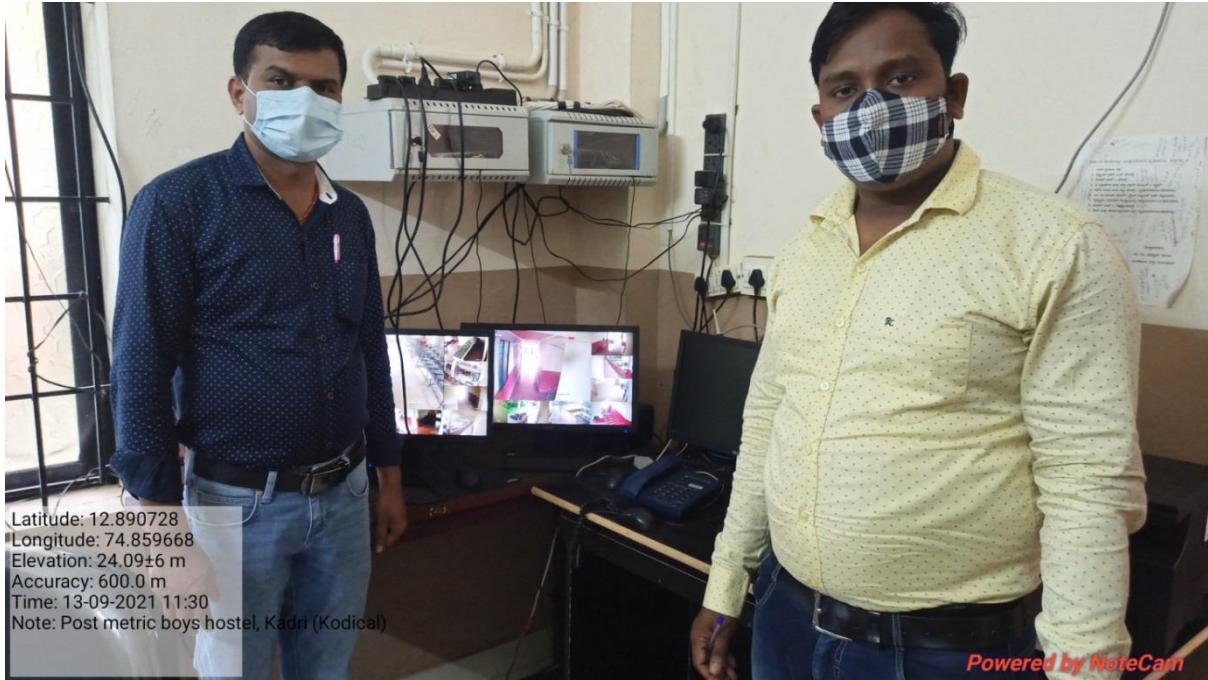
Provision of CCTV
